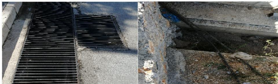
Figure 15: The Drainage System Separating the Rain Water from the Sewage on the Main (Kötekli) Campus
