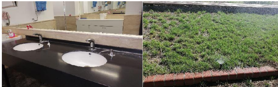
Figure 14: Water Saving Taps and Irrigation System on Campus
